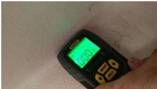
Photo 95-1 Old water stains - 0 percent moisture
