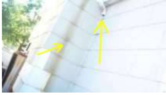
Photo 21-3 Missing downspout - Disregard stain on exterior wall
