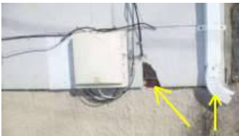
Photo 18-3 Downspout should go to ground level - Disregard Broken Shingle
