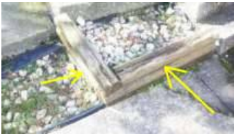
Photo 5-1 Beginning of rotted wood. Also water will sit in this area
