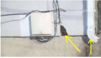
Photo 26-1 Downspout should go to ground level - Disregard Broken Shingle
