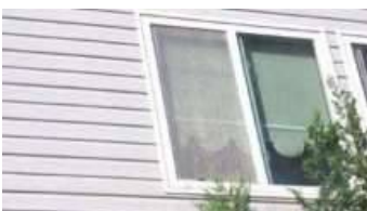
Photo 85-1 Damaged Window Screens
