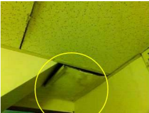
Photo 95-9 Water stain on ceiling tile is from an old leak
