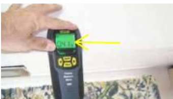
Photo 94-1 47 percent moisture reading
