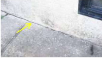
Photo 7-1 Seal this section to prevent water intrusion
