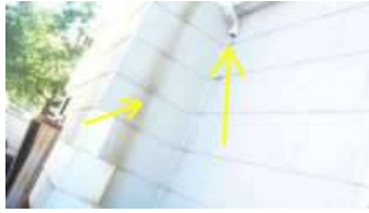
Photo 26-2 Missing downspout - Disregard stain on exterior wall
