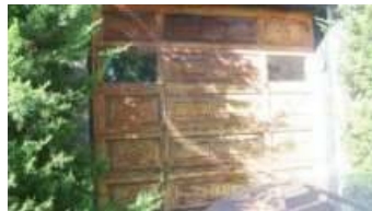
Photo 20-2 Garage door needs refinishing. Was not maintained
