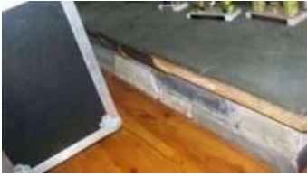
Photo 57-1 Inspectors are not permitted to move items out of way because it is against the Standards of Practice
