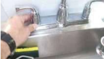
Photo 61-1 Loose kitchen faucet
